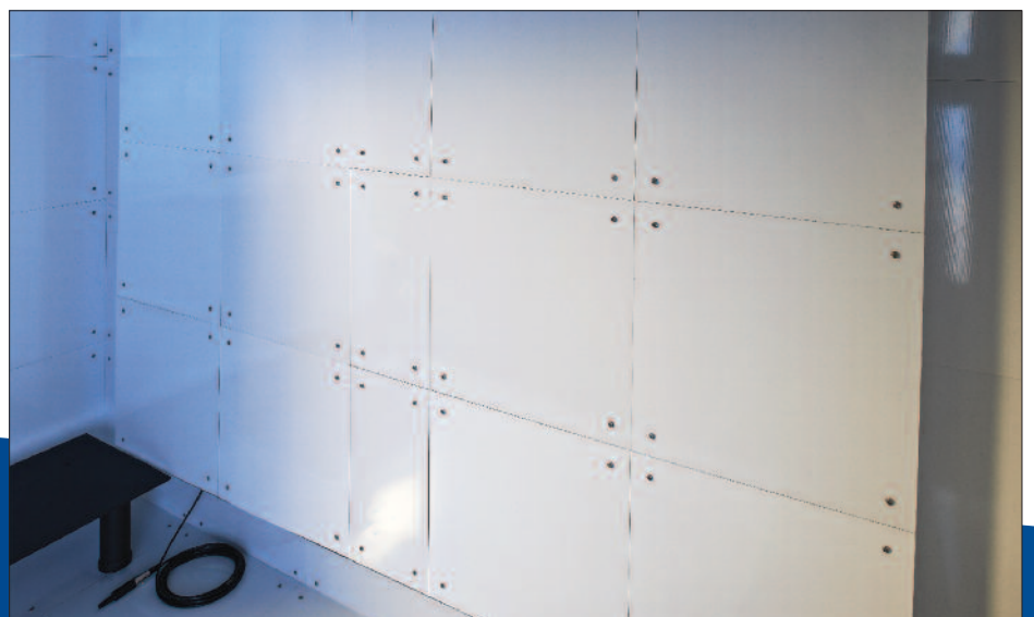
The panels are a close fit to ensure that all of the potential laser exit points are covered.
